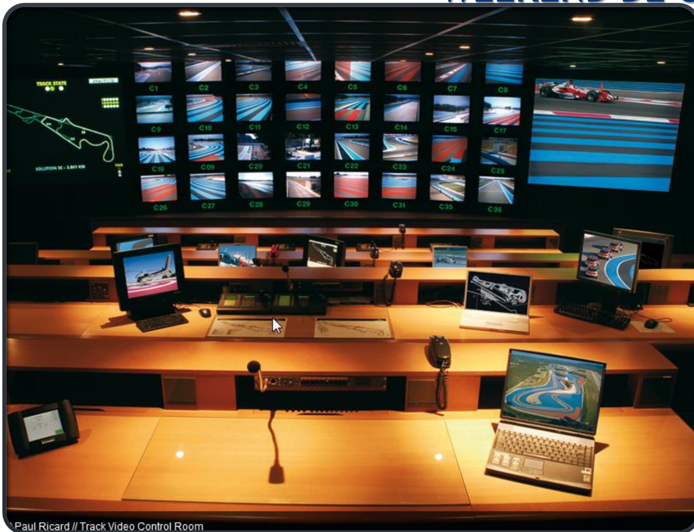
Paul Ricard // Track Video Control Room
